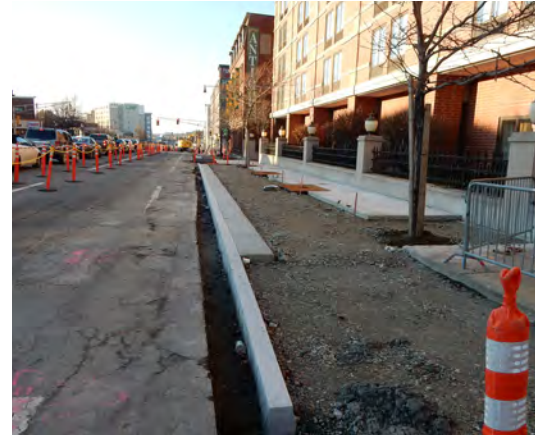
Construction photo of the sidewalk-level separated bike lane on the north side of Route 28 near Water Street (Image looking north west)
